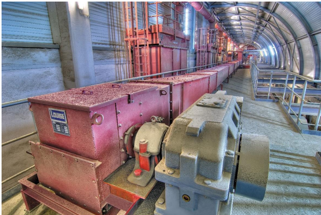
Example application of an AUMUND Drag Chain Conveyor, type LOUISE, in a cement plant (Photo AUMUND)
